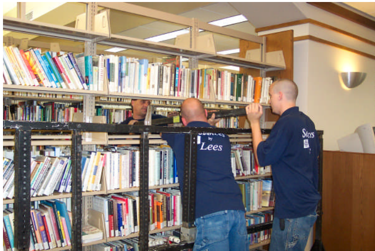
Workers install the LIFT System to raise book shelves so old carpeting may be removed and new flooring installed.
